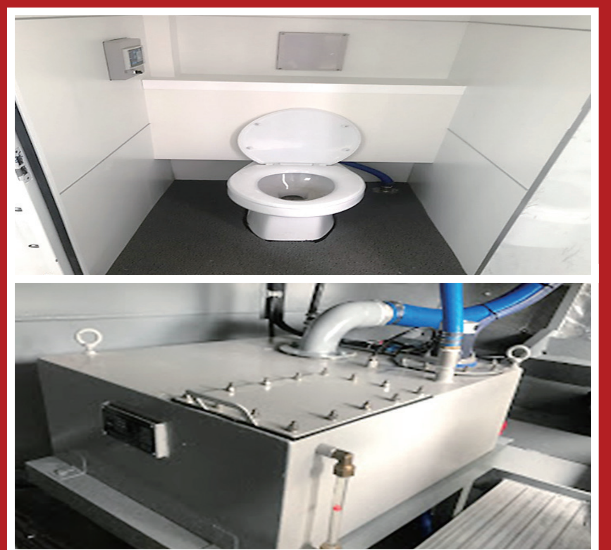
- Nigeria Patrol Vessel sewage comminuting & disinfecting equipment -
